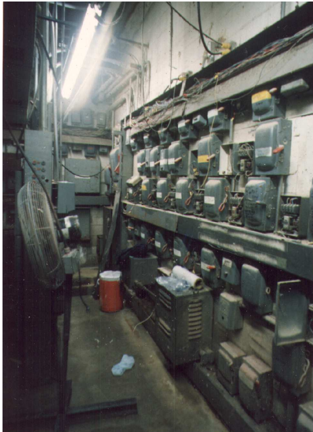
Figure 1 - Existing Electric Room
